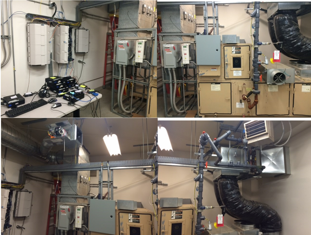
Figure 4.7. Pictures of the HVAC system used for the experiment.
