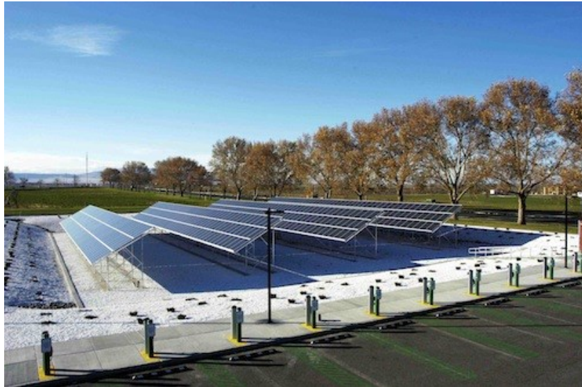
Figure 2.1. Solar PV panels on PNNL campus [source: Hire Electric]
